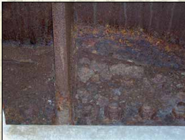
Localized laminar corrosion of weathering steelwork below deck joint (Pre-blast).
