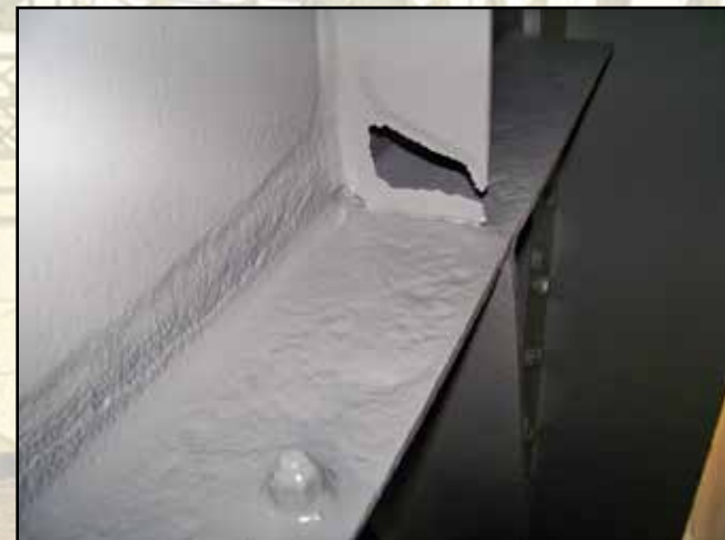
Localized area of 100% section loss and deep pitting uncovered during blasting operations. Painting contract has provisions for repair.
