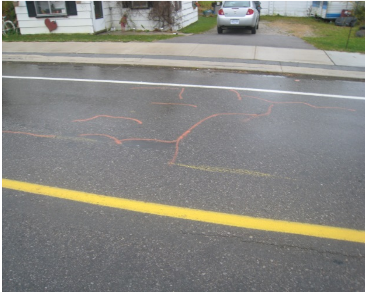
Cracking of new binder course that contained high percentage of RAS
