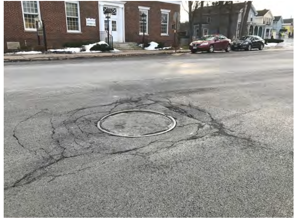
Traditional Frame & Cover Road damage after 2 years
